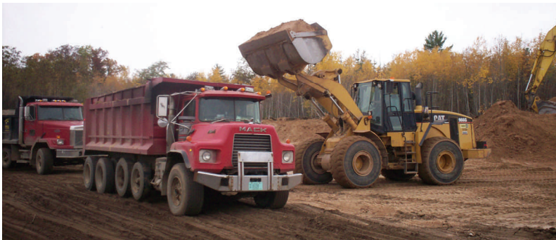
A loader fills a dump truck with sand at Cloverleaf Sand & Gravel. Many loads have been delivered to the substation site on Highway 22.
